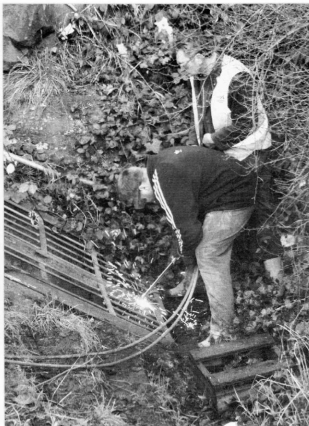
Newcastle City Council workmen cutting the welds of the gate to allow Sub Brit members access to the Group Control Filter Room at Blakelaw
